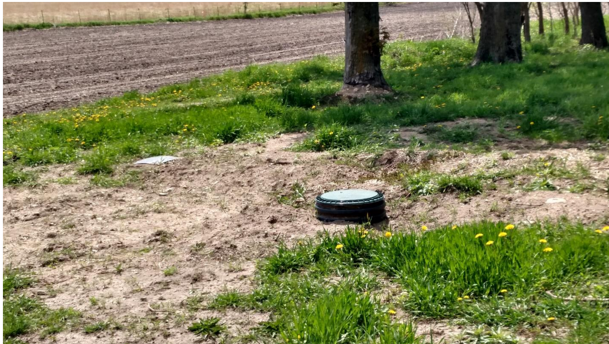
Figure 3 Septic system on the south side of the house
