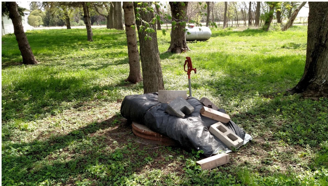
Figure 4 Well on the northwest side of the house
