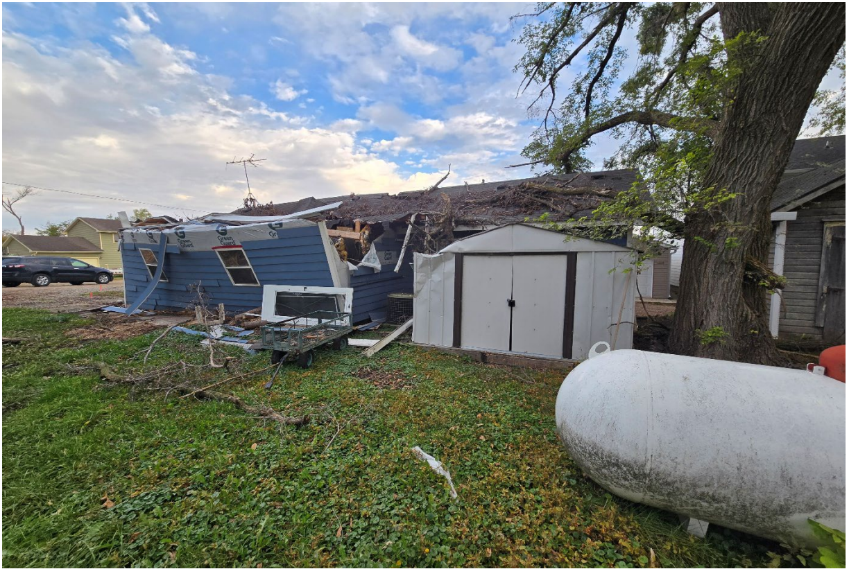
Figure 2 - Storm damage to existing cabin
