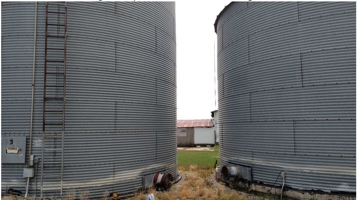
Figure 4 Looking at the separation between the two center grain bins
