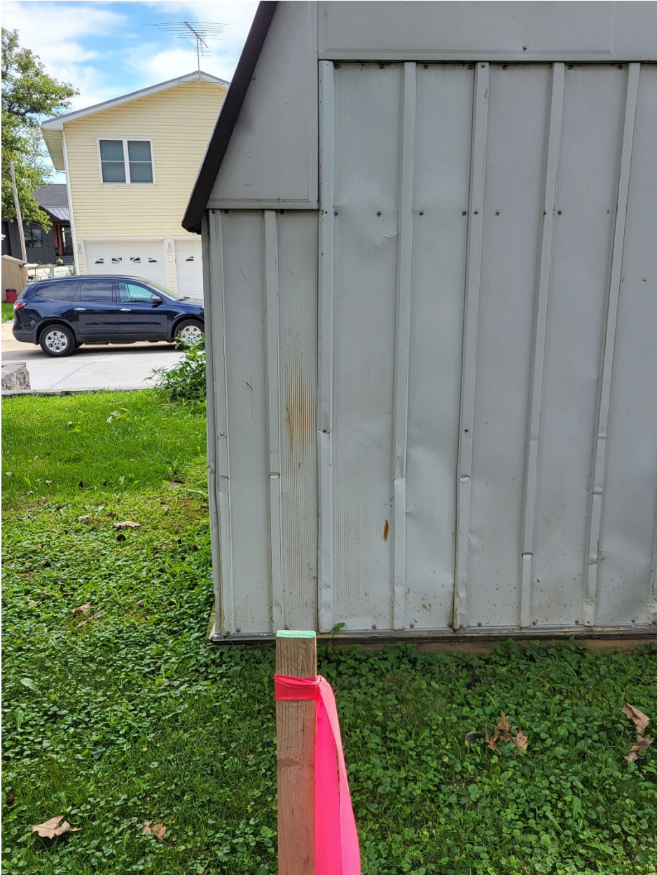
Figure 2 – Looking at encroachment along west lot line from the rear of the property
