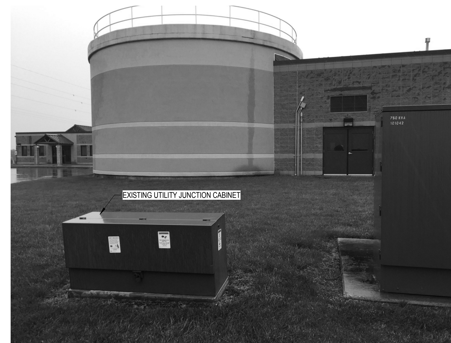
3 EXISTING ELECTRIC UTILITY EQUIPMENT WEST OF DIGESTER BUILDING NO SCALE
